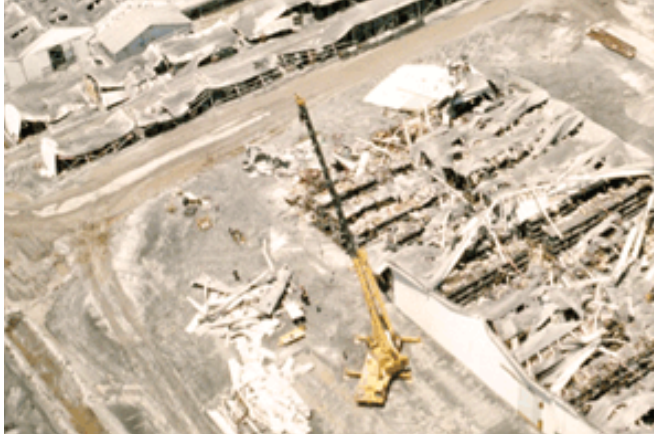
With a force of 62.7 pounds per square foot, the wet volcanic ash collapsed the roofs of countless buildings at Cubi Point and Subic Bay, including this one at the naval station, July 8, 1991. With torches, hand tools and front-end loaders, Seabees dismantled and demolished some structures and repaired the roofs of others. Photo from U.S. Navy Source: https://seabeemagazine.navylive.dodlive.mil/2018/06/15/kicking-ash-the-seabees-of-operation-fiery-vigil/
