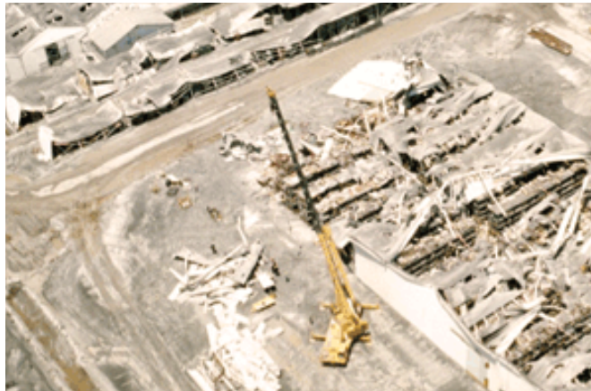
With a force of 62.7 pounds per square foot, the wet volcanic ash collapsed the roofs of countless buildings at Cubi Point and Subic Bay, including this one at the naval station, July 8, 1991. With torches, hand tools and front-end loaders, Seabees dismantled and demolished some structures and repaired the roofs of others.
